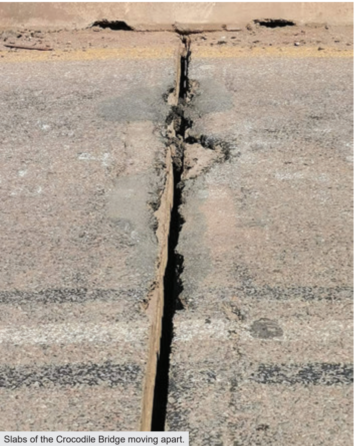
Slabs of the Crocodile Bridge moving apart.
